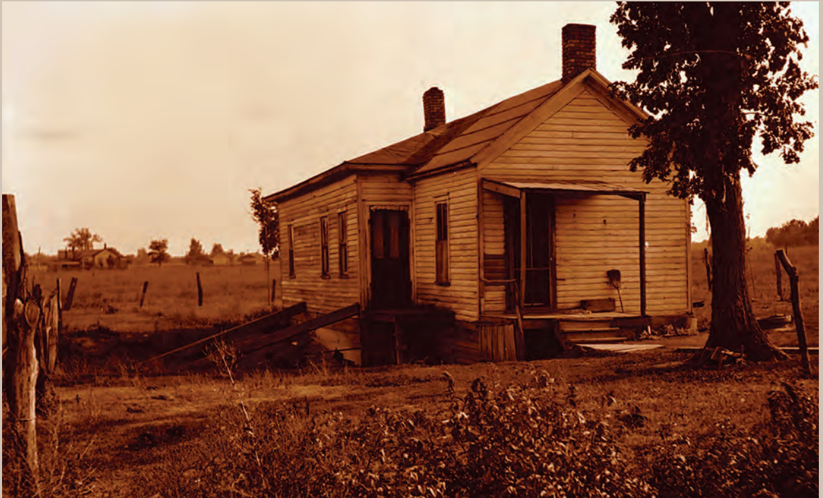
Pit subsidence (10 x 20 ft. wide, 5 ft. deep) which occurred next to a house near Streator, IL. ISGS files/ 1916 Cooperative Coal Mining Series Bulletin 17, Surface Subsidence in Illinois
