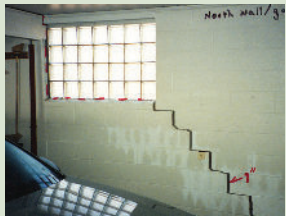
Step cracks, such as these, are not uncommon in block walls affected by mine subsidence.
