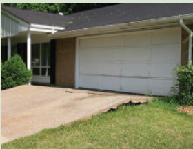
Ground movement from mine subsidence causes this driveway to buckle.
