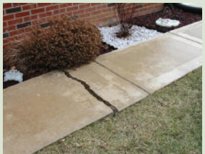
This sidewalk is literally pulled apart by mine subsidence.
