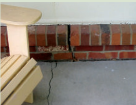
Mine Subsidence can cause cracks in pavement or foundations, as shown above.
