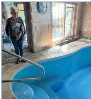
IMSIF CEO Heidi Weber examines cracks in the floor of the indoor swimming pool.
