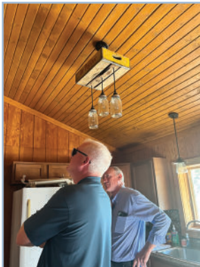
Chairman Rich Sauget and Board member Paul O'Grady examine damage to a structure.
